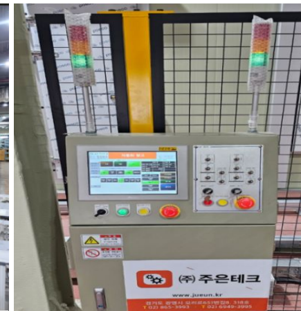
-25 degree refrigerated automatic warehouse STC ground control panel
