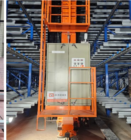
-25 degree refrigerated automatic warehouse
