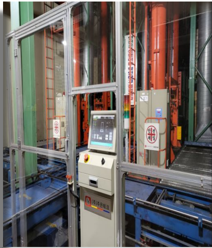
Rack Build' PLT Type automatic warehouse
