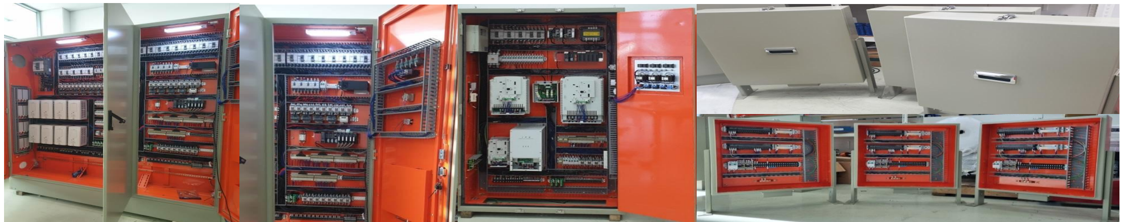
PLC Control Panel Inside
